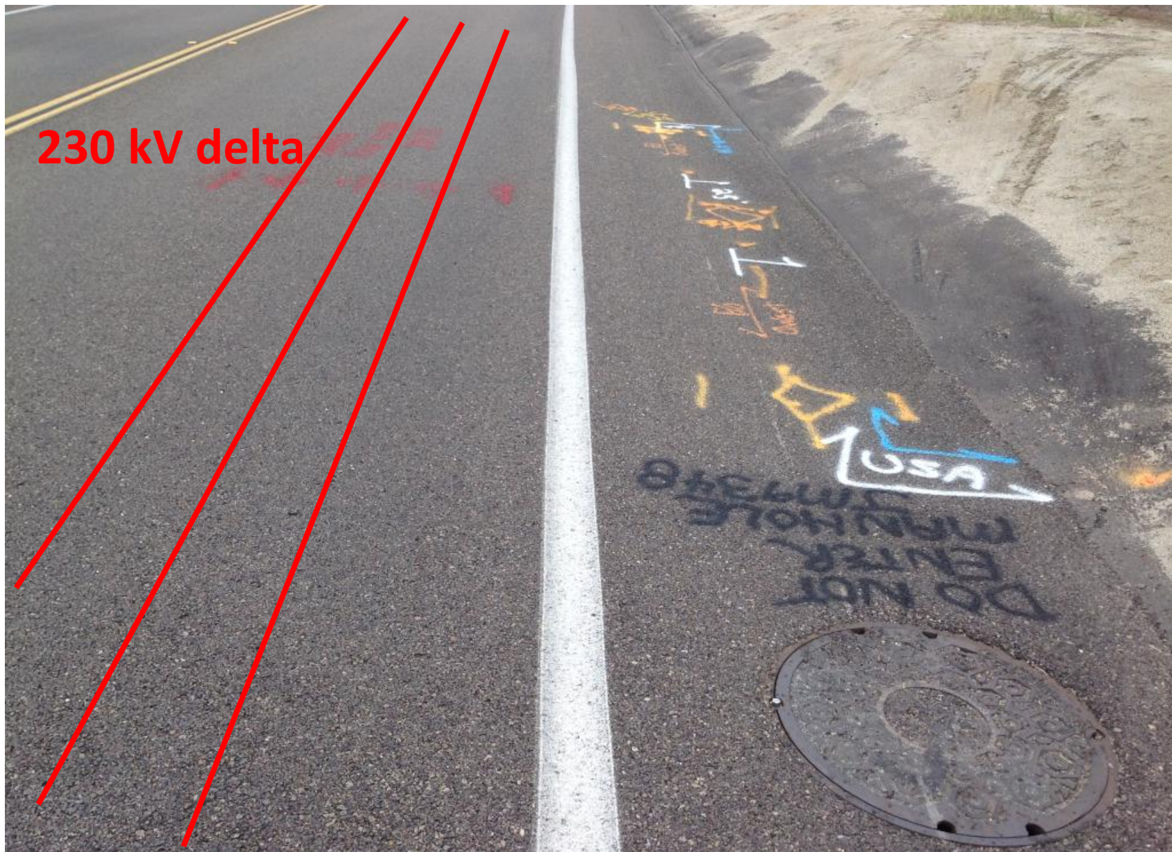
Underground HV transmission line and communications cable
