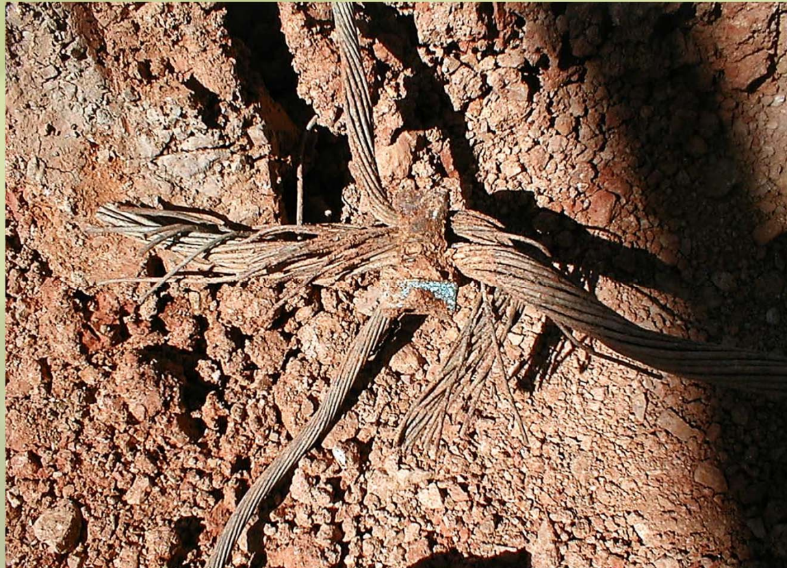
Buried Split Bolt Connection: Guaranteed to last!
