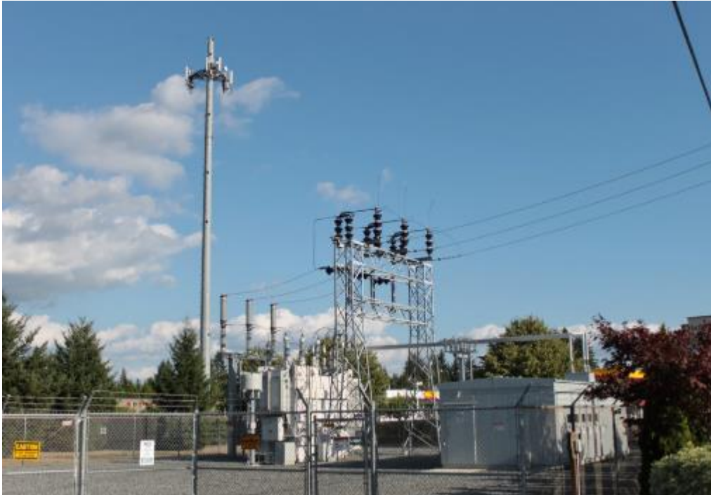
Cell tower in close vicinity to an electrical substation
