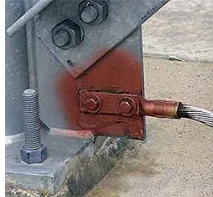
Tinned 4/0 copper conductor attached to a galvanized steel flange of a support column. Note the high pressure compression fitting and protective paint
