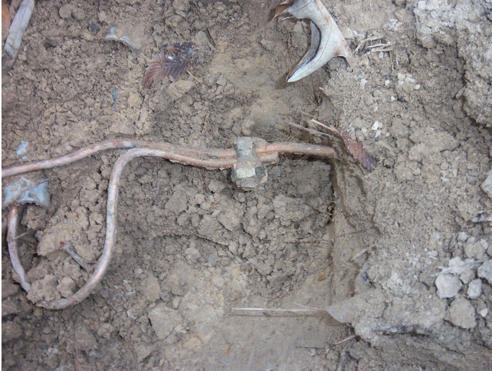
Split bolt used to connect remote cabinet to ground ring.
