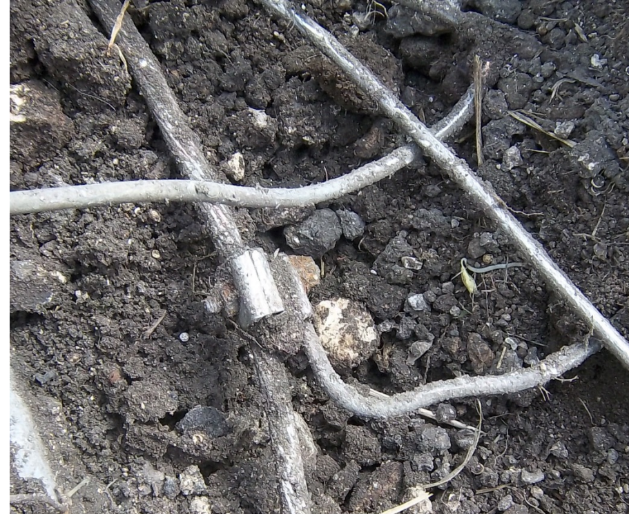
Lashing wire clamp used to connect waveguide ground bar to tower ground ring.
