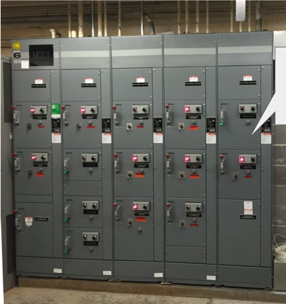
Traditional Motor Control Center
