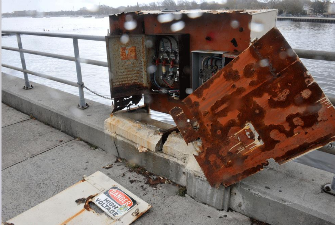
Hurricane damaged electrical equipment cabinet
