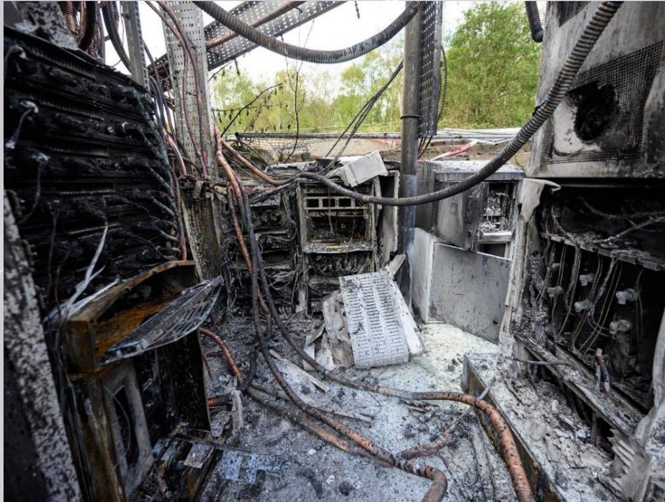
Burned telecom equipment cabinet
