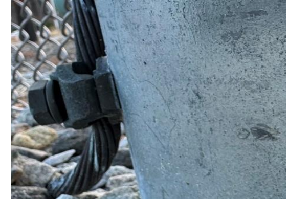
Bare copper connector designed for flat surface installed incorrectly on a round steel pipe
